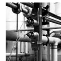
Installation in highly corrosive environment
