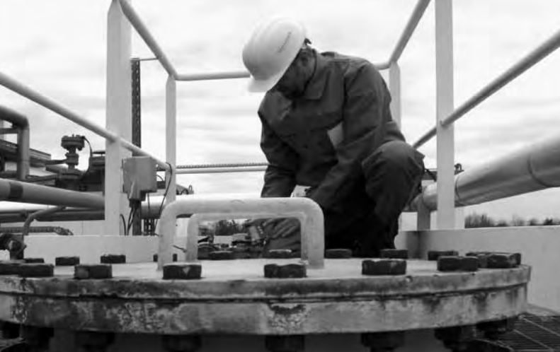
Commissioning of two Micropilot M
