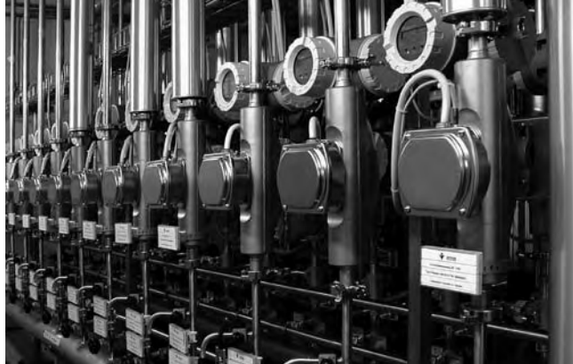
Mass flowmeters mounted vertically
