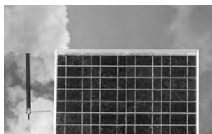
GSM antenna on a solar panel
